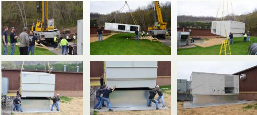
An overhead crane was needed to maneuver the new air handler unit into position for installation
