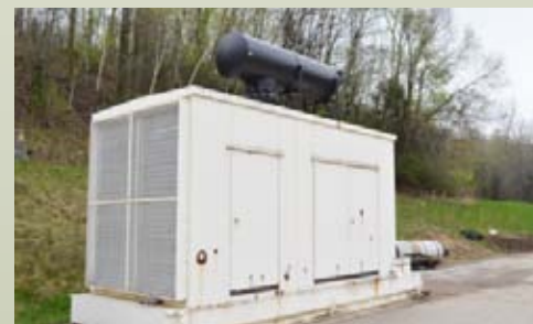
An EPA compliant exhaust system is now in place
